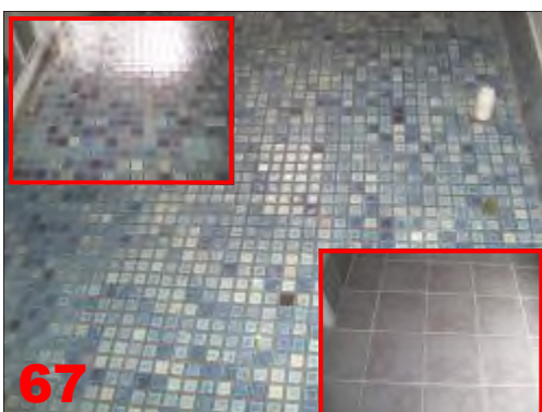
The tile floor finishes showed no excessive lifting or cracking at the time of inspection. (See photo no. 67)
